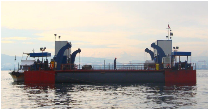
Figure 23: Bedding Preparations for Osmangazi Suspension Bridge Caissons - Kaptan Aydemir Catamaran Type, ULE Carrier Barge (ULE in Operational Position). Courtesy of STFA Construction Co
