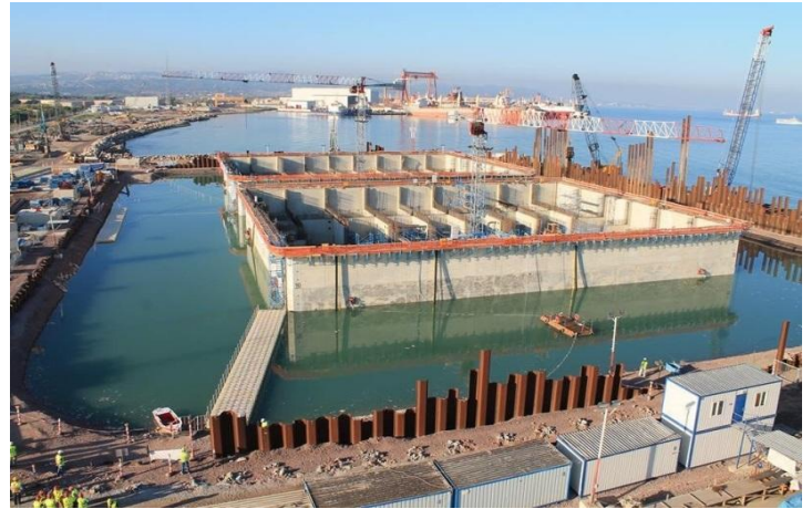
Figure 144: South TF Caisson Floated, Moored at North TF and submerged to the bottom of the Dry Dock temporarily. Courtesy of STFA Construction Co.
