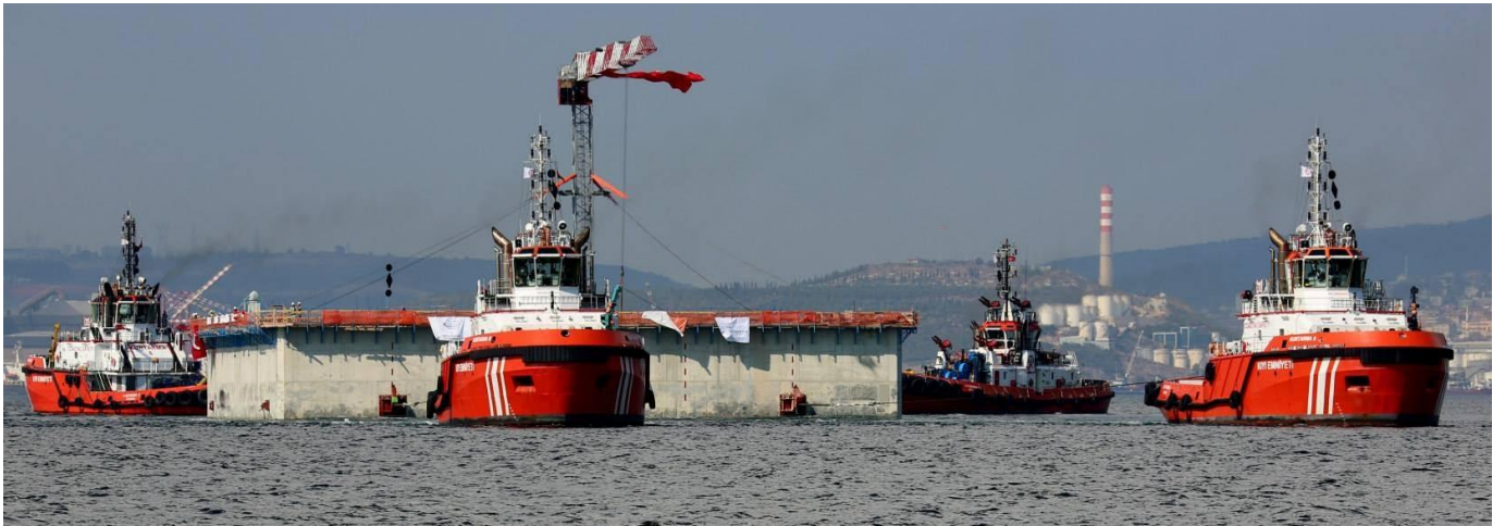
Figure 103: Initial Launching; KURTARMA-9 and KURTARMA-10 are (front) towing the South TF Caisson and KURTARMA-8 and KURTARMA-5 as Trailing Tug Boat. Courtesy of STFA Construction Co.
