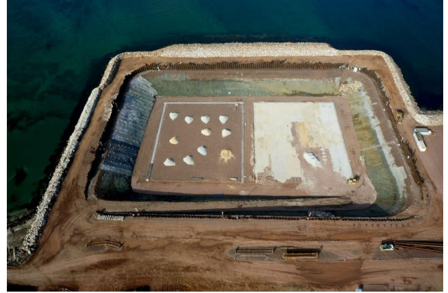
Figure 141: Preparation of the base of the Dry Dock for GBS Caisson Construction. Courtesy of STFA Construction Co.
