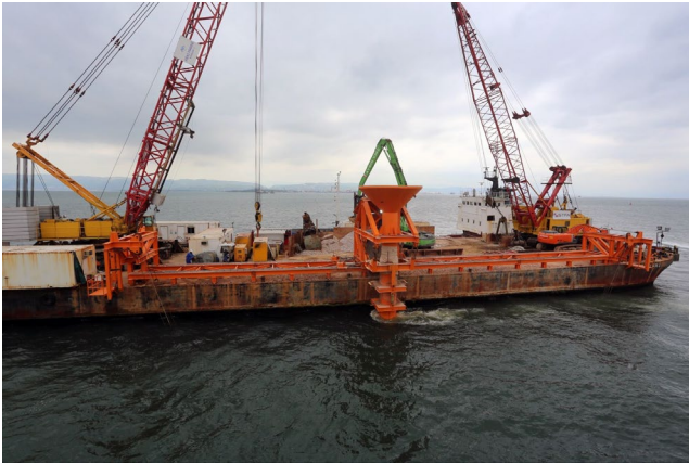
Figure 152: Anti-Scour Rock Placement - Filter Layer (Crushed Stone) by Fall Pipe Barge. Courtesy of STFA Construction Co.
