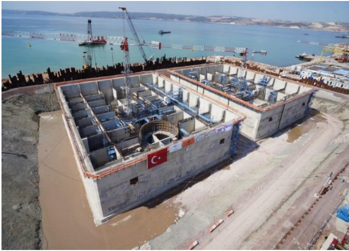
Figure 143: Taking Water to the Dry Dock, after the completion of the Caisson Construction. Courtesy of STFA Construction Co.
