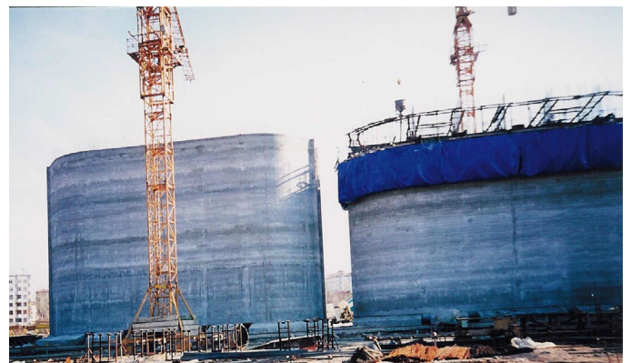
Figure 72: The Caissons under Construction. The blue canvas covers the upper moulds system
