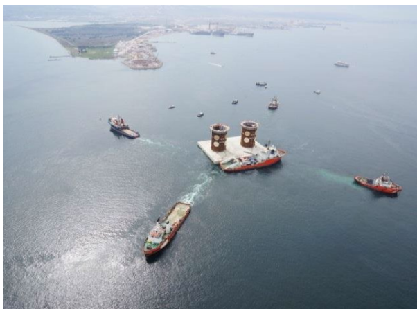
Figure 8: Submerging of Gravity Base Structure GBS Solution (Floating). Courtesy of STFA Construction Co. Osmangazi Suspension Bridge South Tower Foundation 8,9
