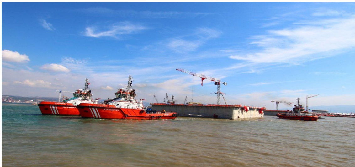
Figure 102: Initial Launching; KURTARMA-9 and KURTARMA-10 are towing the South TF Caisson and KURTARMA-5 is hooking up as Trailing Tug Boat. Behind is Diana-II (STFA's Work Boat) assisting with the Hook-up Operation. Courtesy of STFA Construction Co
