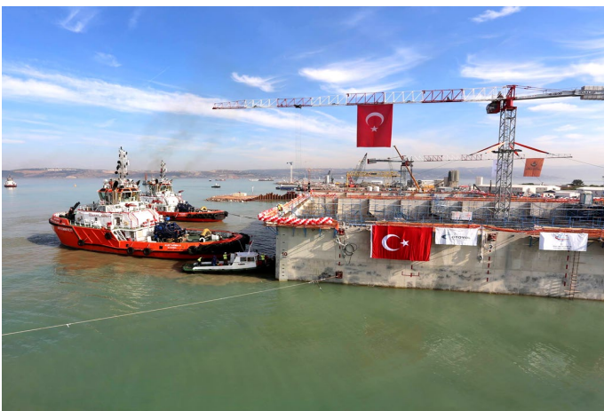
Figure 82: Initial Launching Stage of the Osmangazi Suspension Bridge's South Tower Foundation Caisson. Courtesy of STFA Construction Co.
