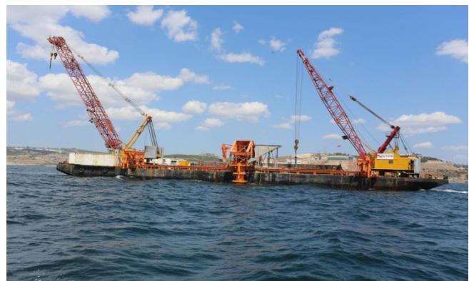
Figure 17: A Fall-Pipe Barge 'Alparslan-2' in operation - Bedding Preparations for Osmangazi Suspension Bridge Caissons. Courtesy of STFA Construction Co.
