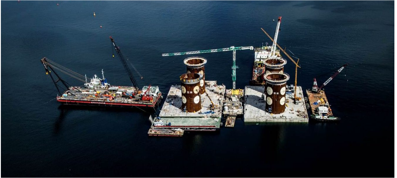
Figure 131: The Caissons are ready to Hook-Up and Tow at Wet Dock. Courtesy of STFA Construction Co.
