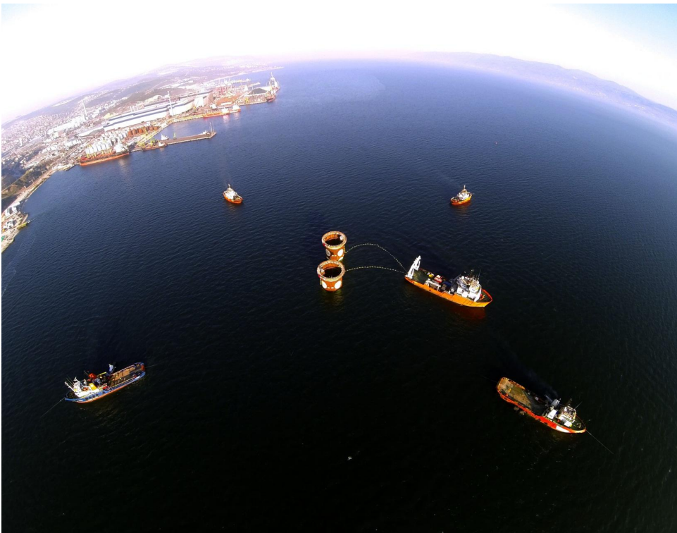
Figure 134: Installation / Submerging of Caisson at the North Tower Foundation Location. Courtesy of STFA Construction Co.
