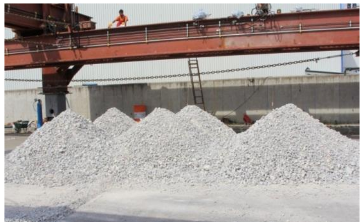
← ↑ Figures 20 and 21: Bedding Preparations for Osmangazi Suspension Bridge Caissons - the Land Tests of ULE. Courtesy of STFA Construction Co.
