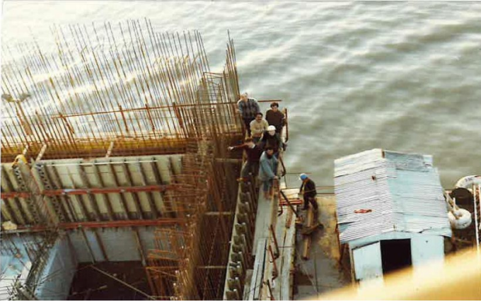
Figure 46: A view of The Marmara Ereğlisi LNG Terminal Caisson from the Construction Stage on the Ocean Going Submersible Barge of STFA (Koca Yusuf-II). Courtesy of STFA Construction Co.(from CEng. Mr. Arif Yeşiltepe's Private Archive)
