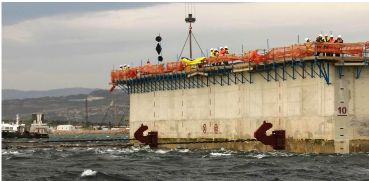
Figure 104: Initial Launching of North TF Caisson, on the left is 'ServetKaradağ' (STFA's Assisting Tug Boat). Courtesy of STFA Construction Co.
