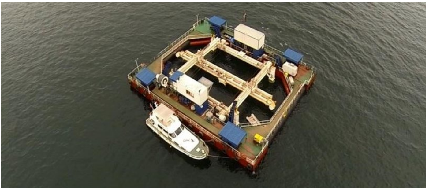
Figure 24: Bedding Preparations for Osmangazi Suspension Bridge Caissons - ULE at Stand-By Position on Kaptan Aydemir Barge. Courtesy of STFA Construction Co.
