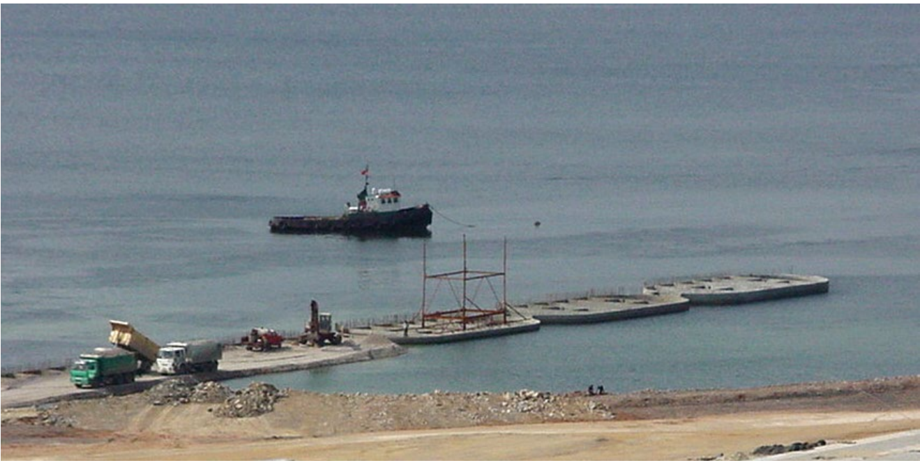
Figure 54: A view of The Belde Port Facilities Quay Wall Construction Project. Courtesy of STFA Construction Co.
