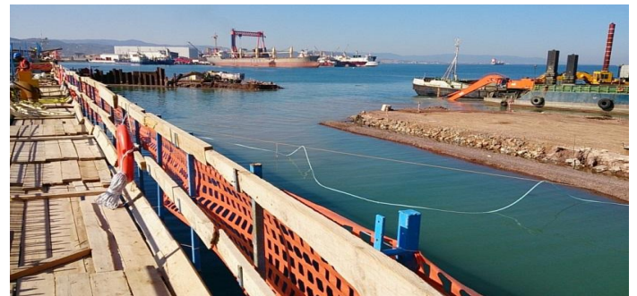
Figure 145: Removal of the Sheet Pile Cofferdam and Temporary West Bund. Courtesy of STFA Construction Co.
