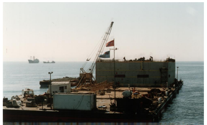
Figure 50: The Water Intake Caisson cast on Submersible Barge (STFA's Koca Yusuf II) at Marmara Ereğlisi LNG Terminal, just before the submerging operation. Courtesy of STFA Construction Co.
