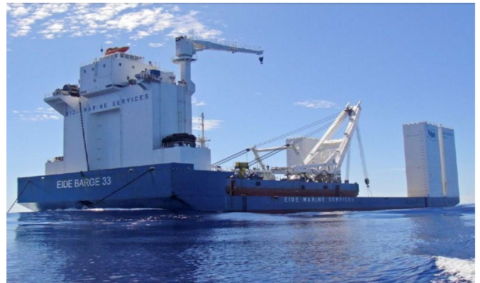
Figure 135: 8,000-ton Caissons are cast by Portal Crane Combined Slipform Method of BYGGING-UDDEMANN AB and Submersible Barge – Eide Barge 33 (Operated by STFA-SGTM JV) is to receive caisson for lowering it to the Sea. Courtesy of STFA Construction Co.
