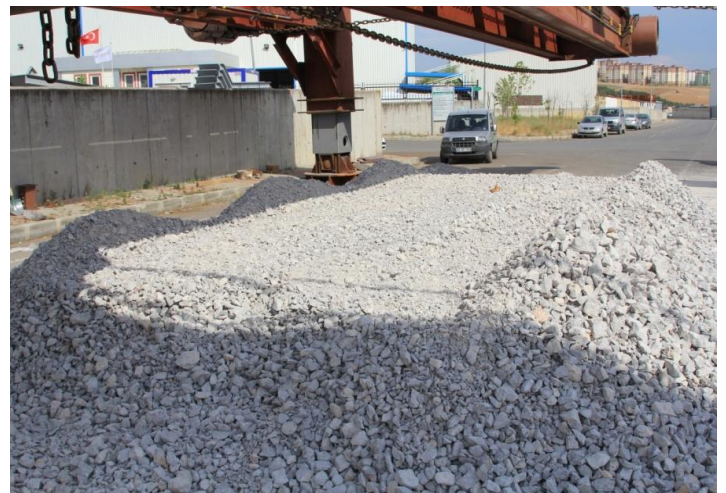
Figure 22: Bedding Preparations for Osmangazi Suspension Bridge Caissons - the Land Tests of ULE. Courtesy of STFA Construction Co.
