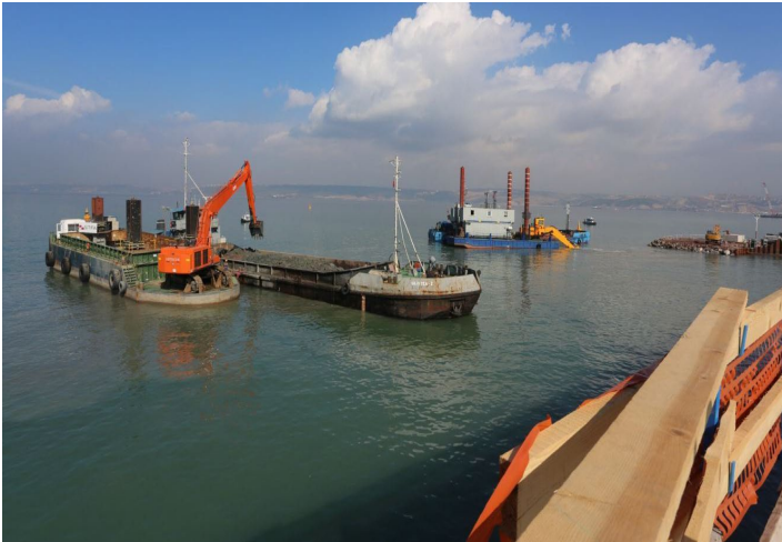
Figure 16: Dredging using Back-Hoe Deeper Dredger, Osmangazi Suspension Bridge Approach Channel Dredging. Courtesy of STFA Construction Co.
