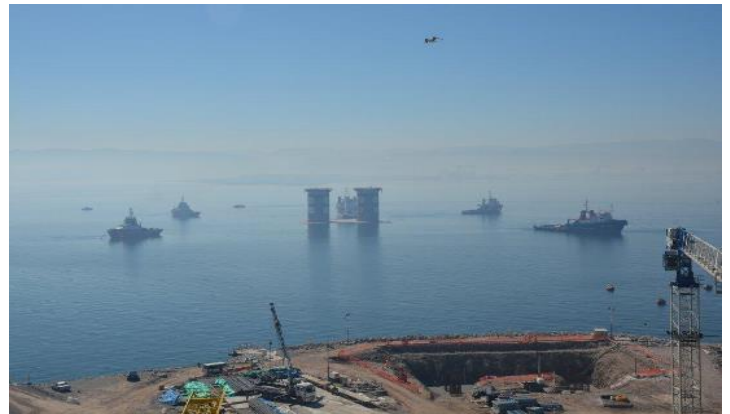
Figure 133: Installation Scheme; Installation Vessels are Moored to Anchor Legs which are previously installed by the means of 'YaşarDoğu-I' (STFA's AHT) Guard / Hook-up Vessel at North TF and DSV (DP2 Diving Supply Vessel) 'SPS Astrea' (Behind the Caisson) is located at its planned position to control to Submersion Operation.
