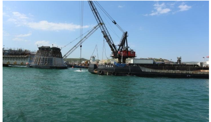
Figure 153: Anti-Scour Rock Placement by Grab-equipped Floating Crane. Courtesy of STFA Construction Co.
